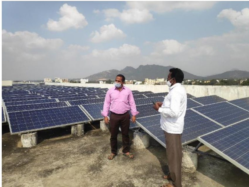
Visit to Solar Power plant in East Block
